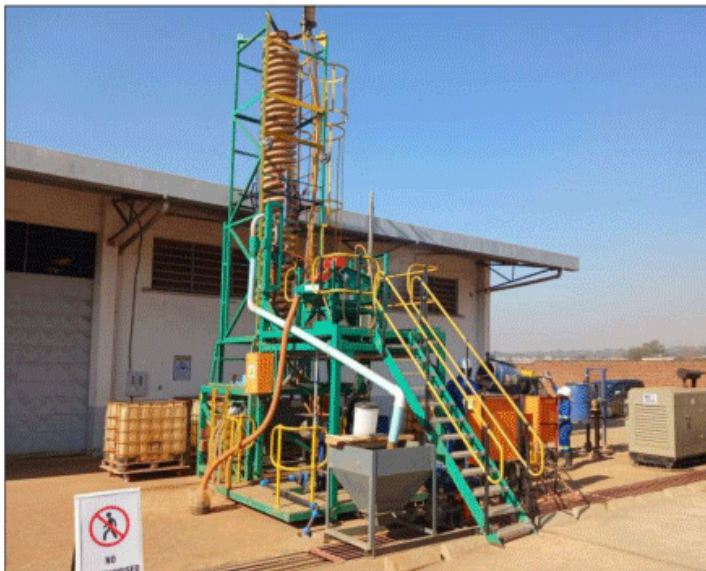
Figure 1: Installed Spiral plant at Sovereign's Lilongwe facility
