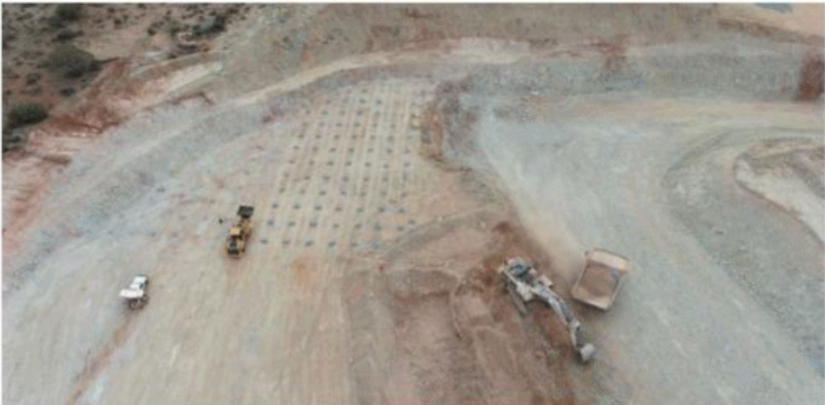
Plates 1 to 3 from top: view looking NW, Stage 1 West Lode mining, view of drill blast pattern (bottom)
